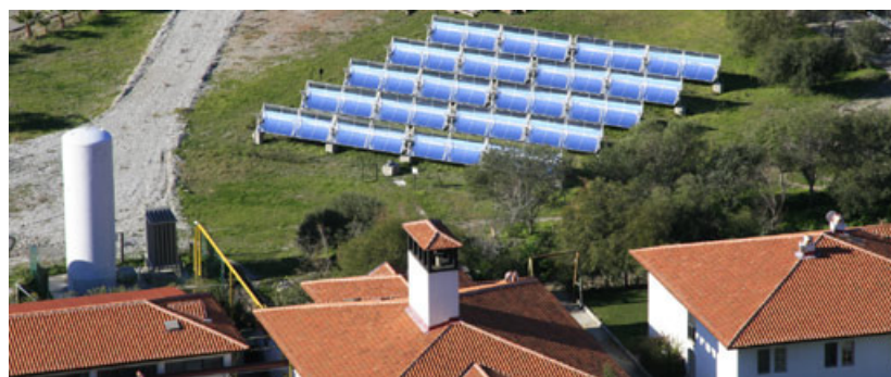
Parabolic trough collectors supplying a hotel in Turkey with process steam for solar cooling and the hotel laundry. Courtesy: MAN Ferrostaal AG; de Riese
