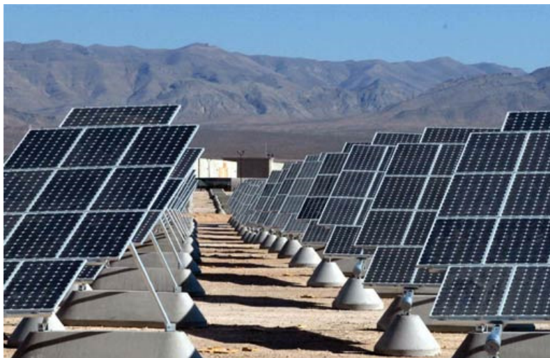
Photovoltaik-Kraftwerk in den USA. Quelle: Greentech Media Research.
