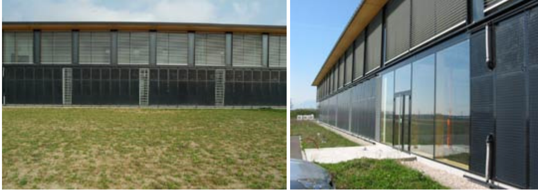
Solar façade with non-glazed stainless steel collectors (in the pictures bottom left and right in the foreground). Photos: Energie Solaire S.A.
