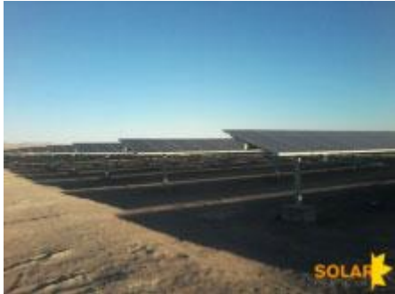
Solarpacks Photovoltaik-Kraftwerk Pozo Almonte I in Chile
